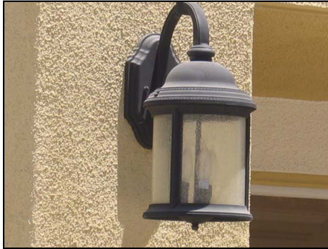
Exterior Light Fixture
